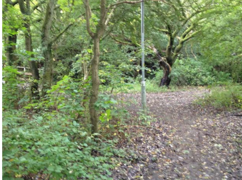
Lighting column to be inspected and repaired or replaced as required
